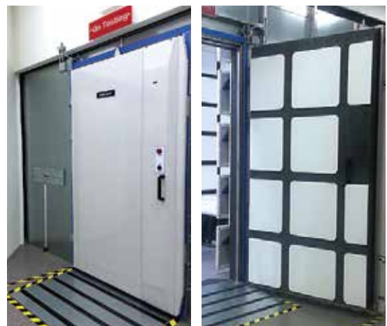
Security Card System & Inside View mounted Absorbers
